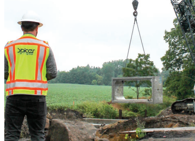
Crews installed larger culverts to accommodate the flow in the John Earl Drain.
