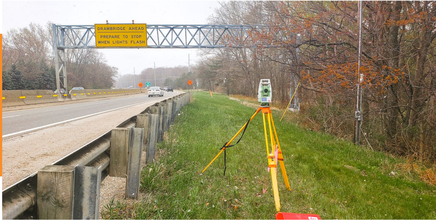
Looking south down US-31 as survey crews begin to map with a Leica total station.
