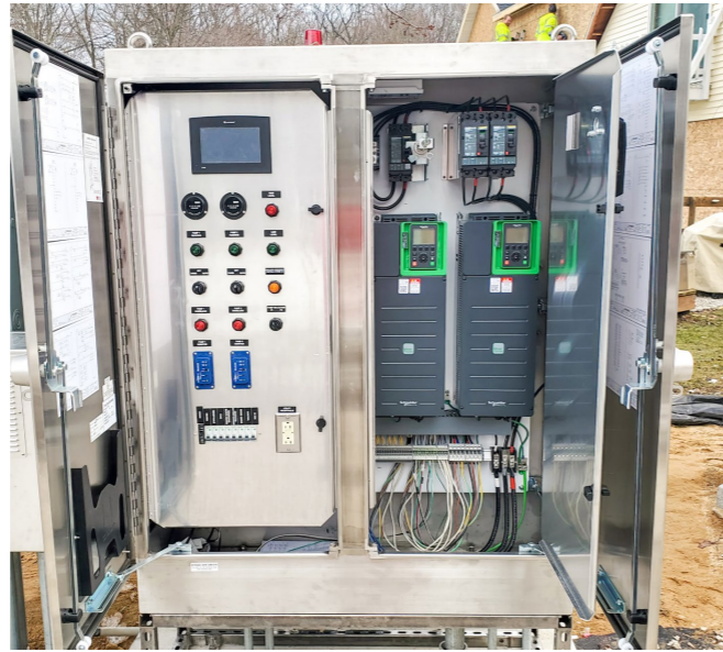
Updated pump station controls.
