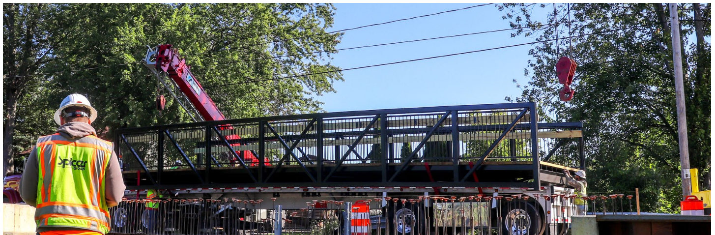
Construction Engineer, Jeff Lentz, oversees the installation of a pedestrian bridge on the Iosco Exploration Trail.
