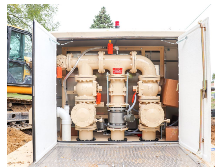
Interior view of above-ground sanitary sewer pump station.
