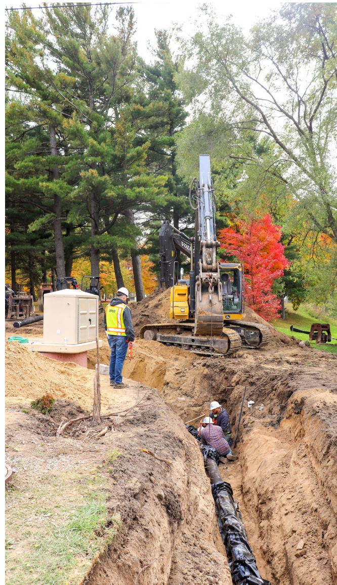
Sam Szaroletta, P.E., inspecting the contractor bolting up a fitting on the new force main.
