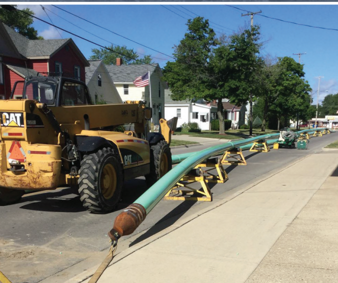
Above: New force main pipe waiting to be pulled under the Manistee River.
