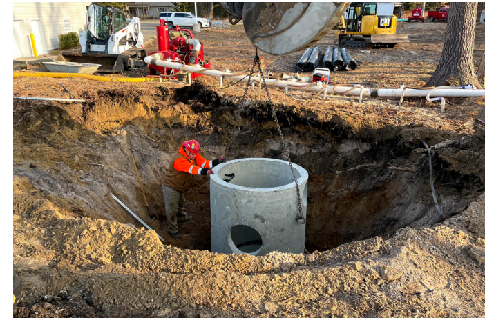
A manhole structure being installed west of Retreat Drive for storm sewer infrastructure that connects detention ponds to the Beechtree Drain.
