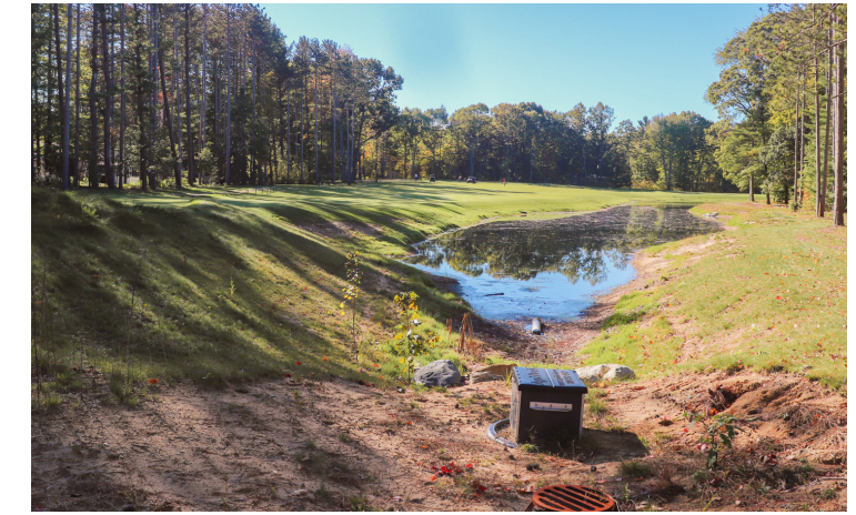
Water level control structures were installed as a part of the Beechtree Drain Improvement Project to allow the OCWRC to efficiently control storm water storage and flow along the drain.
